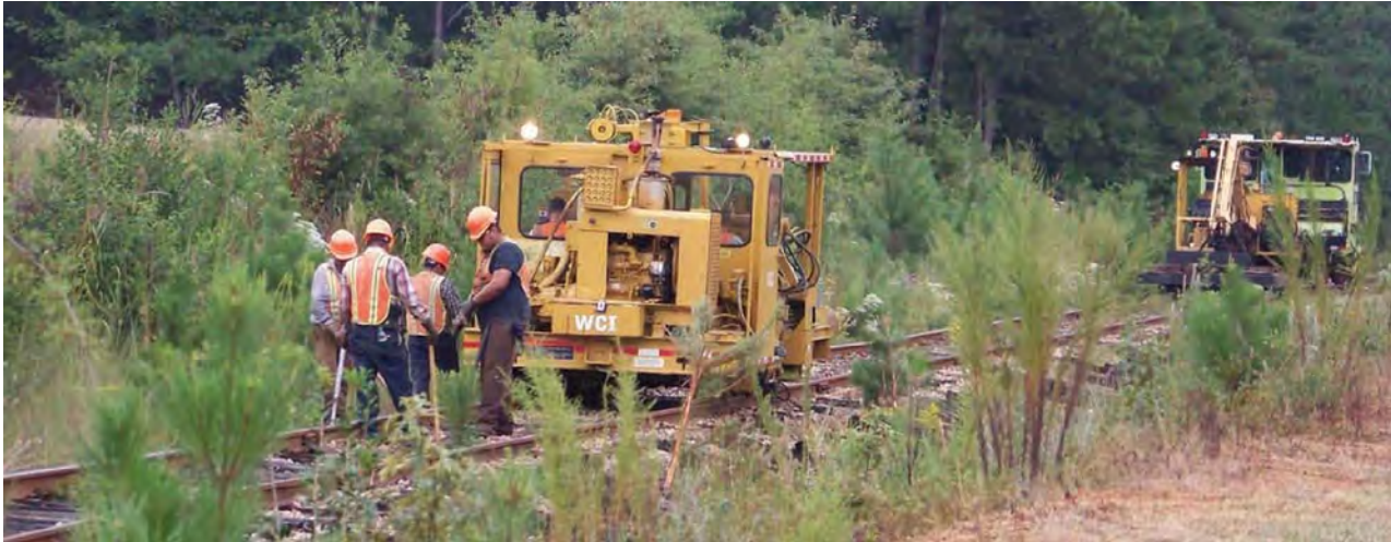
South Carolina-based Wilson Contractor, Inc., handles major track work for Greenville & Western.
